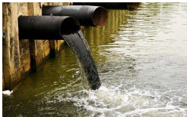
Polluted wastewater being disposed to natural body of water
